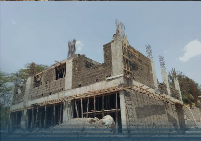
Lower Ground floor- Wing B walling viewed from lower parts of the lot.
